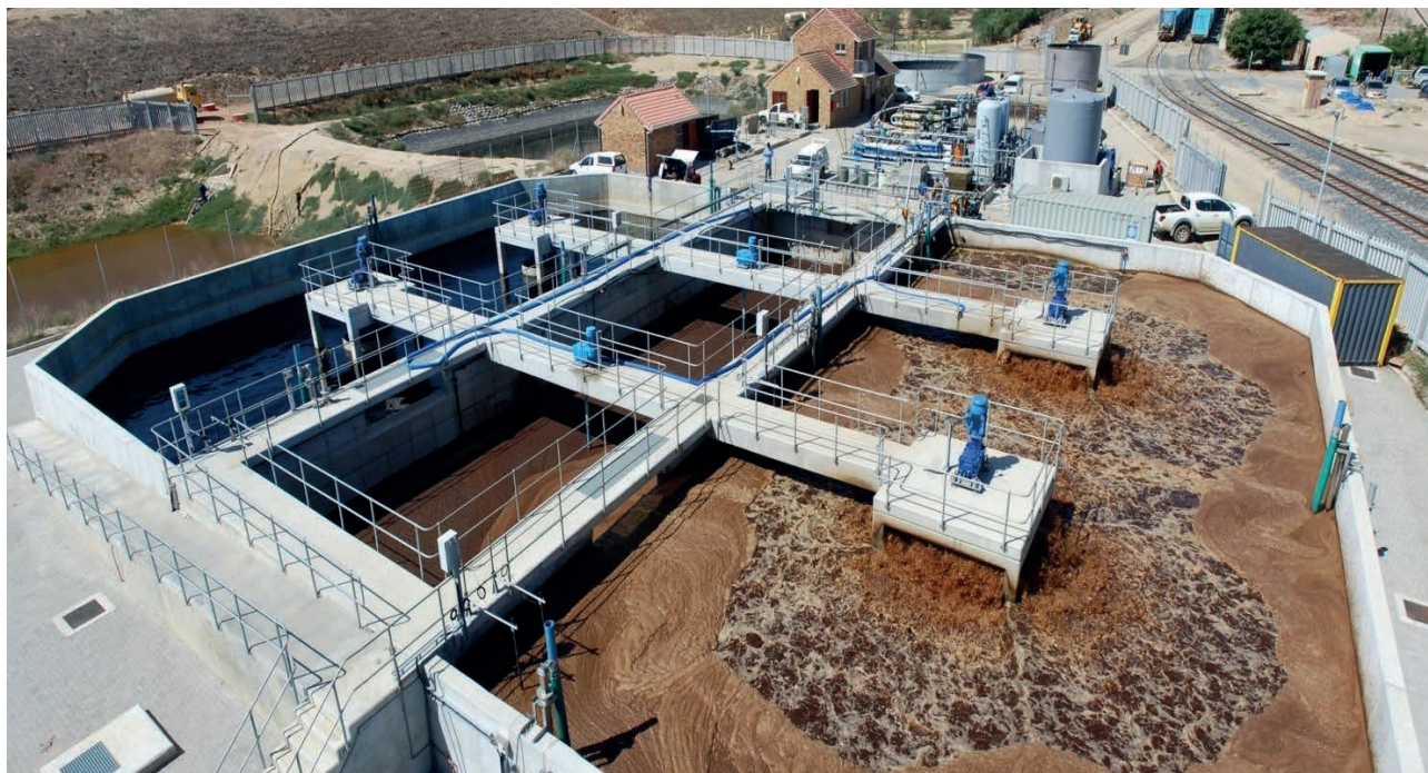
PLATE 1: Vissershok Landfill Leachate Treatment Plant, Cape Town, South Africa.
