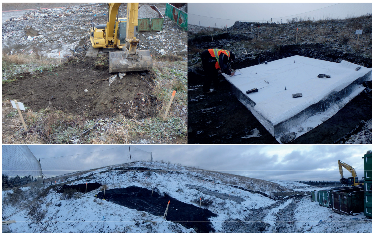
FIGURE 2: Photos showing the cleaning of the surface (top left photo), the measurement of initial ASER (top right photo), and the final appearance after the installation of the cover materials.
