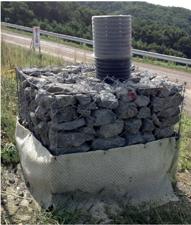
FIGURE 2: A typical landfill gas venting pipe.
