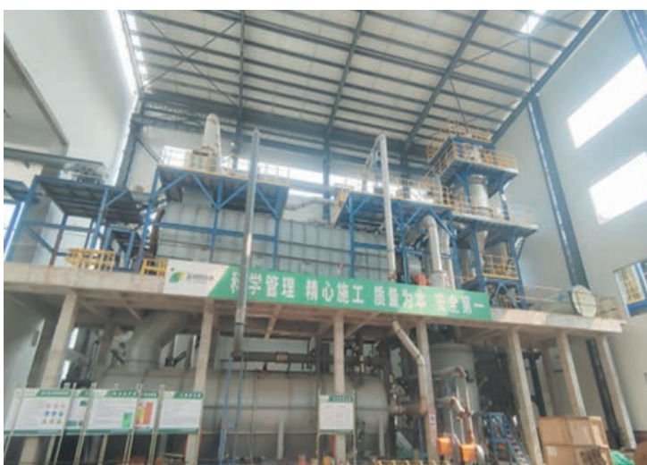
FIGURE 3: Shaoxing Hazardous Waste Center, Zhejiang Province, China (2022). Capacity: 15000 Mg per year (wet basis) of chemical sludge.
