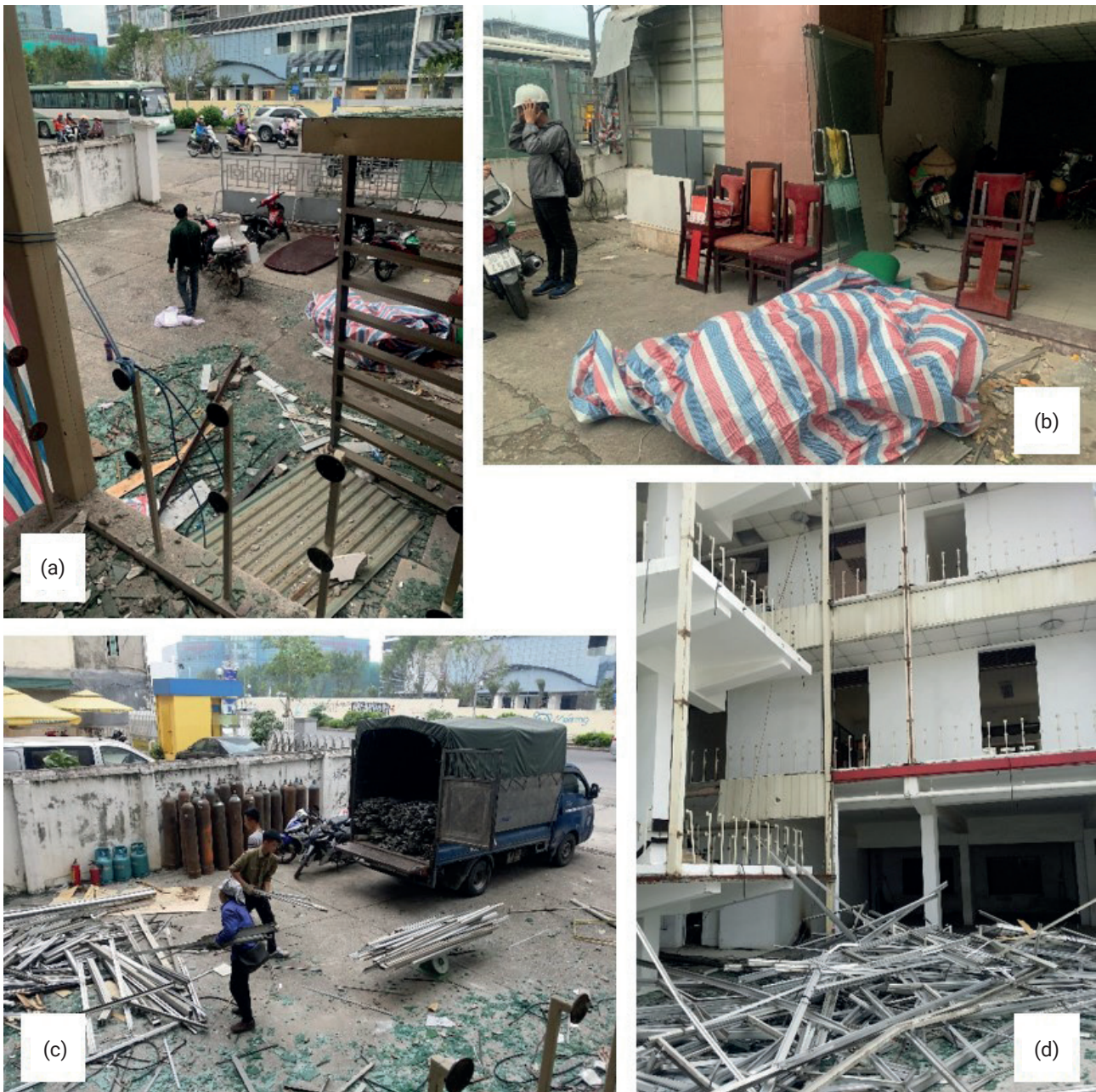
FIGURE 7: Removal of (a) sanitary ware; (b) interior furniture; (c) and (d) aluminum façade at OFC-01.
