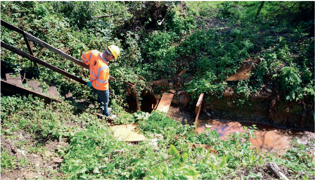
PLATE 2: General view of the more recently installed leachate collection point at the Sump on the Bleakdown landfill site.
