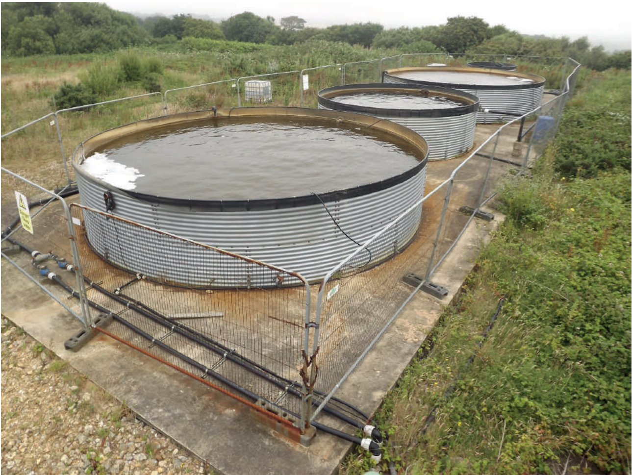
PLATE 4: The Bleakdown landfill leachate treatment plant (LTP) in July 2016, prior to refurbishment work.
