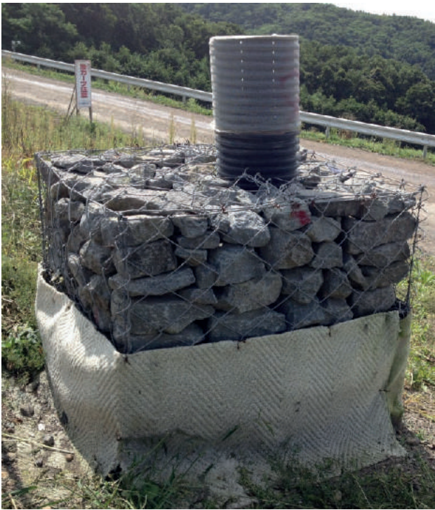
FIGURE 2: A typical landfill gas venting pipe.
