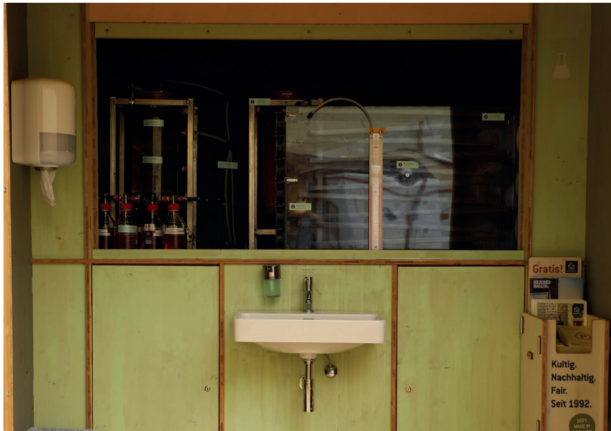
FIGURE 6: Urine treatment units inside the P-BANK.
