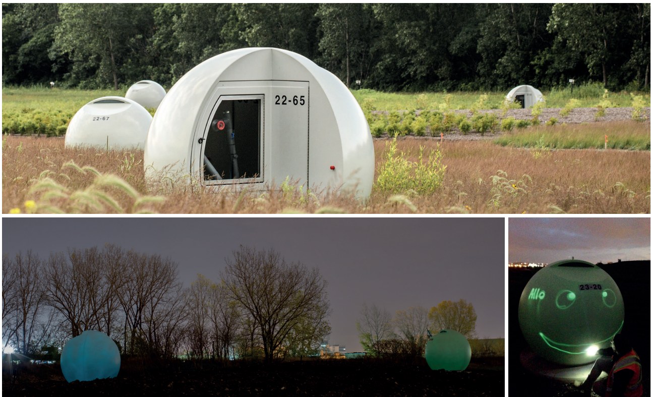
FIGURE 10: The spheres are designed to protect the LFG collection wells and make part of the park experience.
