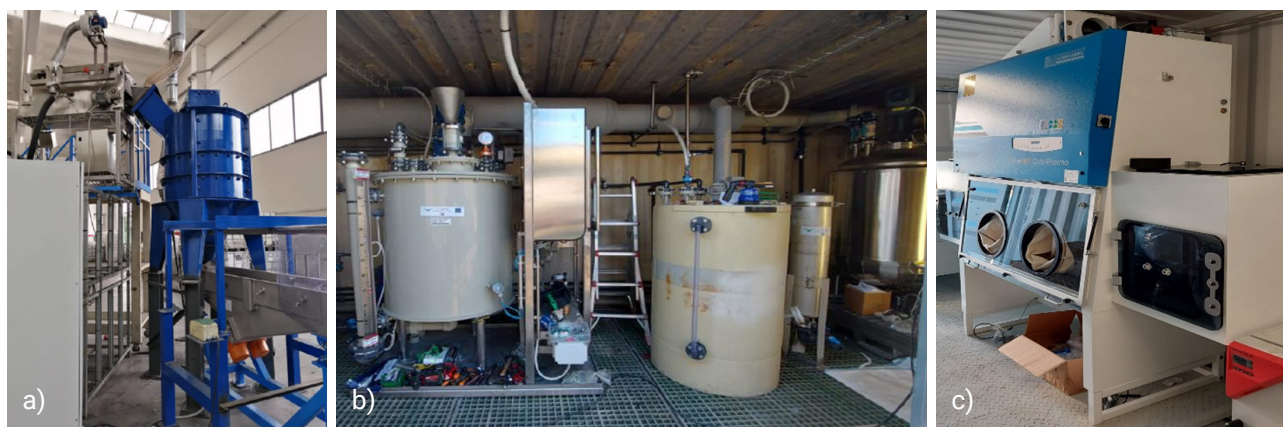
FIGURE 2: Sections of the pilot plants: the cryo-mechanical section (a), the hydrometallurgical section for resynthesis (b), and the cathodic material production section (c).
