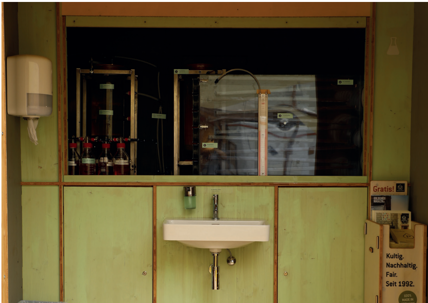
FIGURE 6: Urine treatment units inside the P-BANK.
