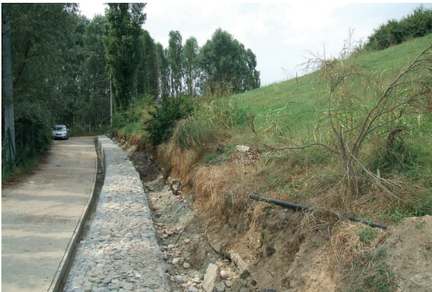
FIGURE 6: After the demolition of the wall, a permeable containment gabion is realized.
