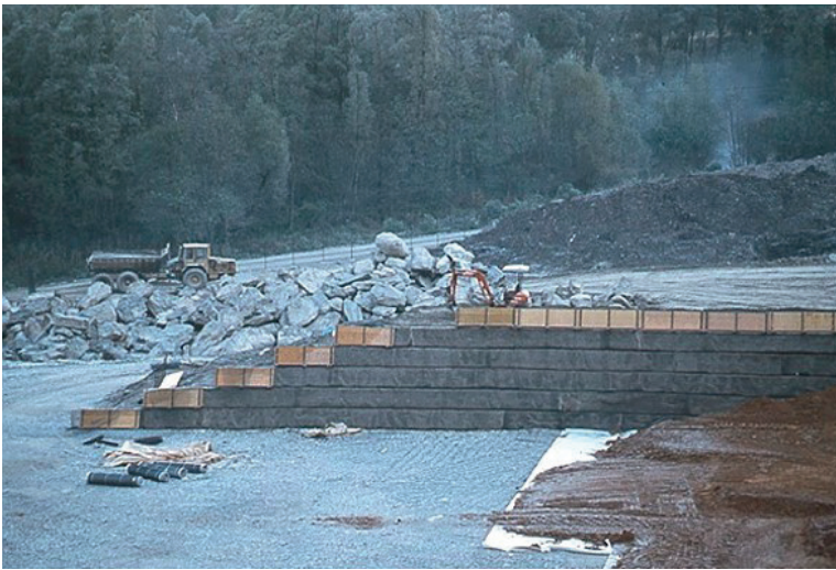
FIGURE 5: Teglio landfill; internal side of the landfill (compacted clay layer can be seen).
