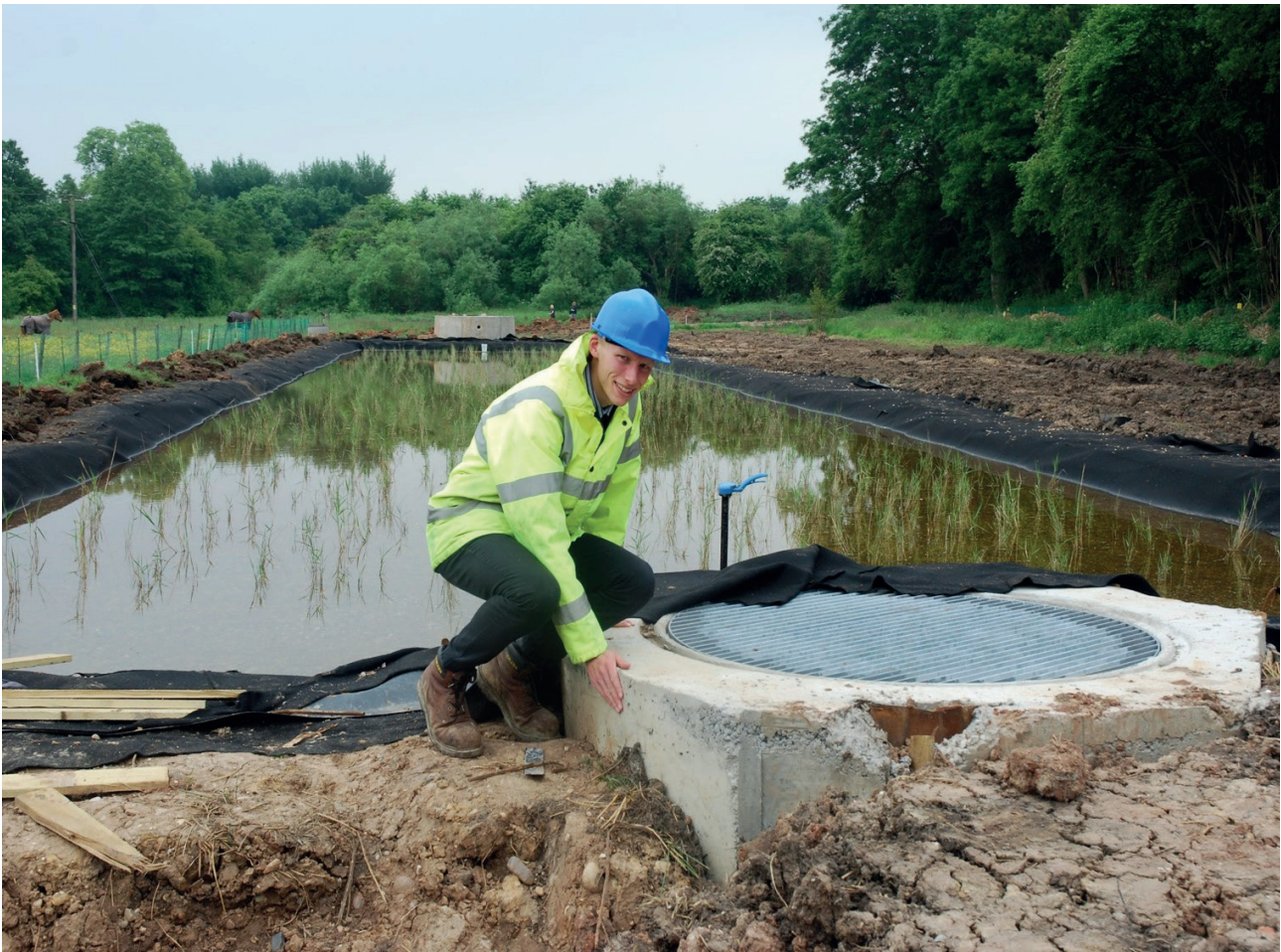
PLATE 1: The chamber at the outlet end of the Shirley Reed Bed during the construction phase of the reed bed
