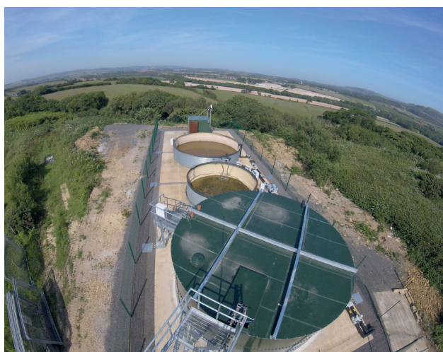
PLATE 5: The Bleakdown landfill leachate treatment plant (LTP) in June 2017, following the refurbishment works.
