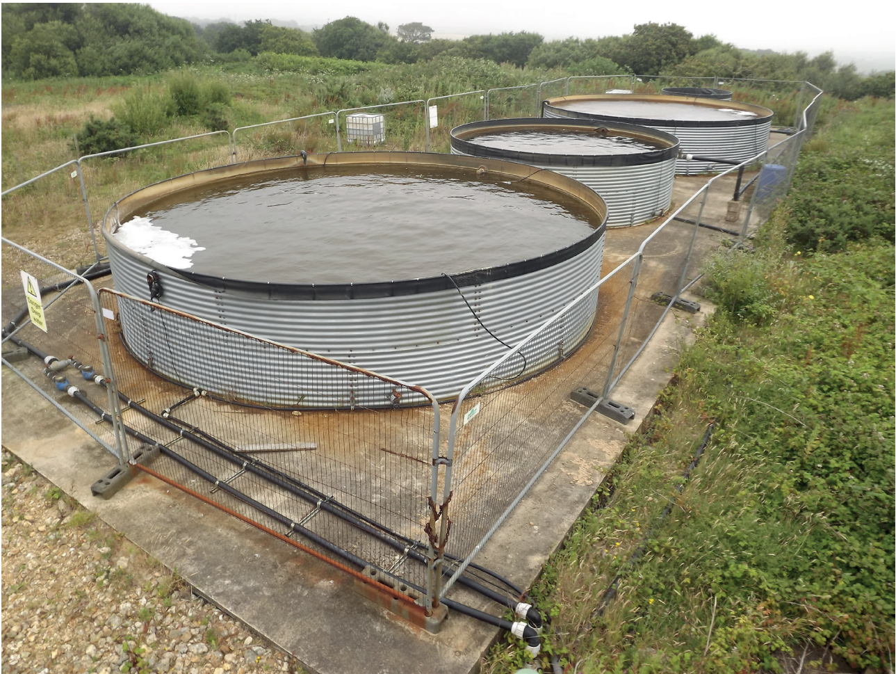
PLATE 4: The Bleakdown landfill leachate treatment plant (LTP) in July 2016, prior to refurbishment work.
