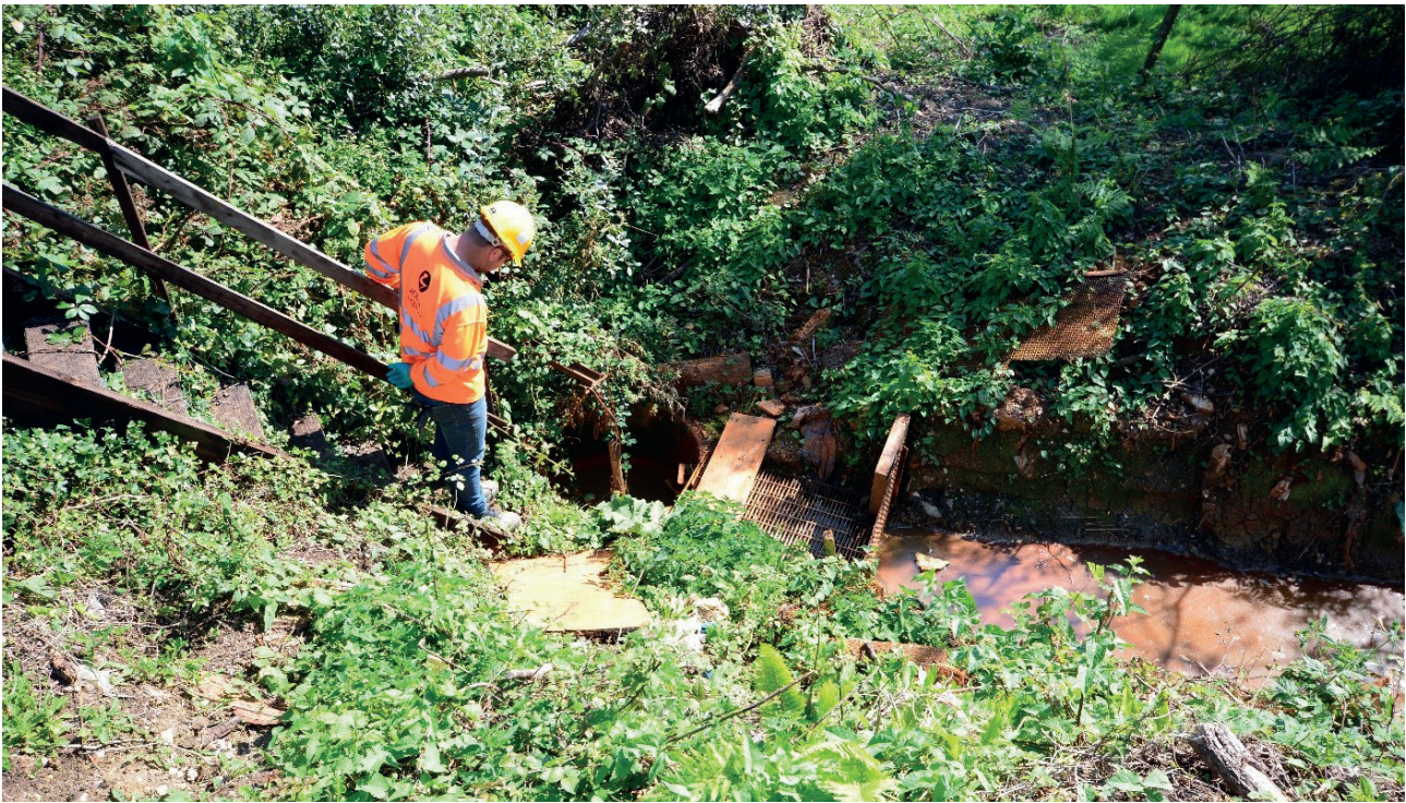
PLATE 2: General view of the more recently installed leachate collection point at the Sump on the Bleakdown landfill site.
