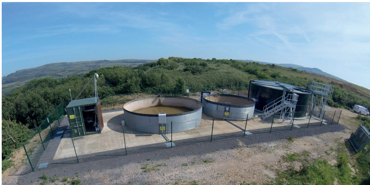
PLATE 1: Aerial photograph of the Bleakdown landfill leachate treatment plant (LTP), showing the control building, RLBT, TLBT, and new glass/epoxy fused steel SBR tank (left to right).
