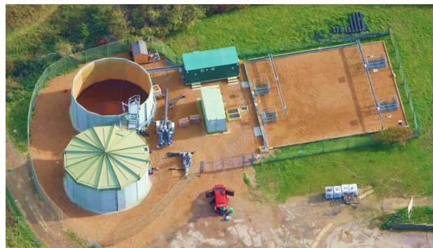
PLATE 1: Aerial view of the updated Leachate Treatment Plant, following modifications made by Phoenix Engineering in 2010.
